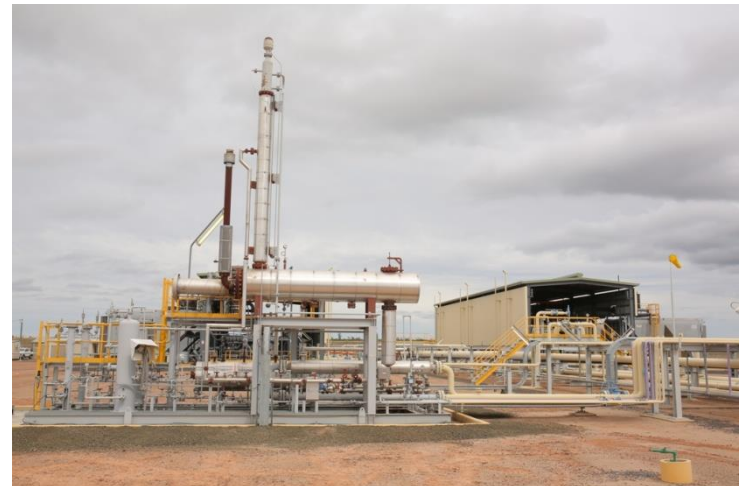
Dalby Tipton | Central Gas Processing Facility
